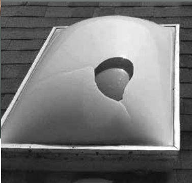
Old acrylic domes can be easily damaged.
